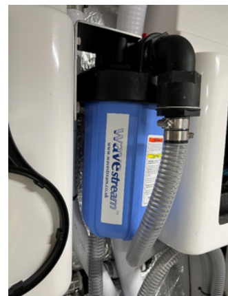
Wavestream System 1 Installation
